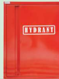
Hydrant Box A2
